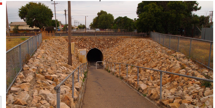
Poor amenity and unsafe pedestrian tunnels
