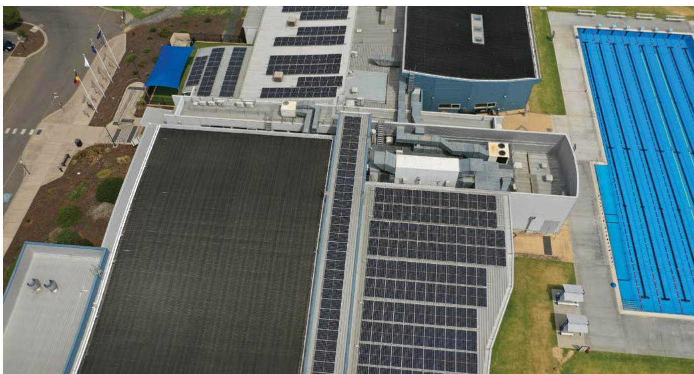
Solar panels were installed on the roof of the Horsham Aquatic Centre and several other Council buildings this year (page 55)
