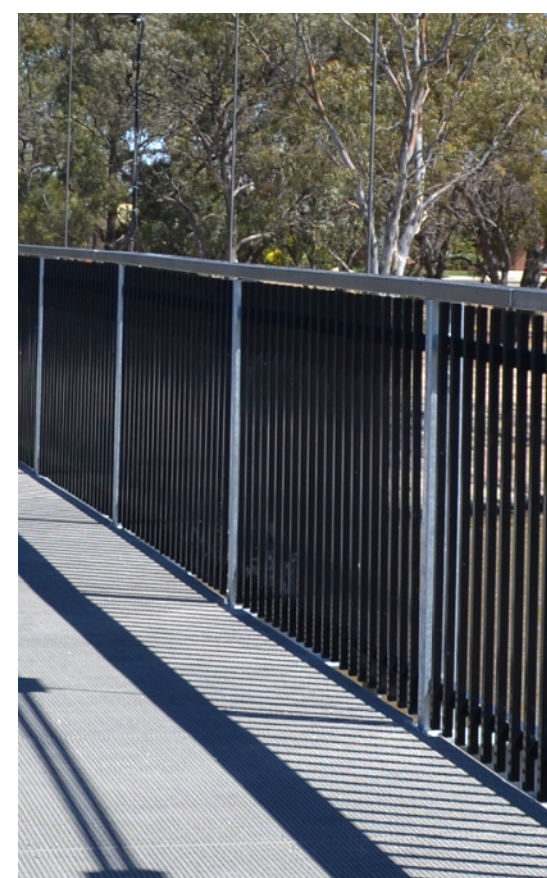
Inspirational Photo: Existing Bridge - micromesh decking with no handrail. Proposed design to have a double handrail and infill to have a flat top (with no neck entrapment) or upper rail.
