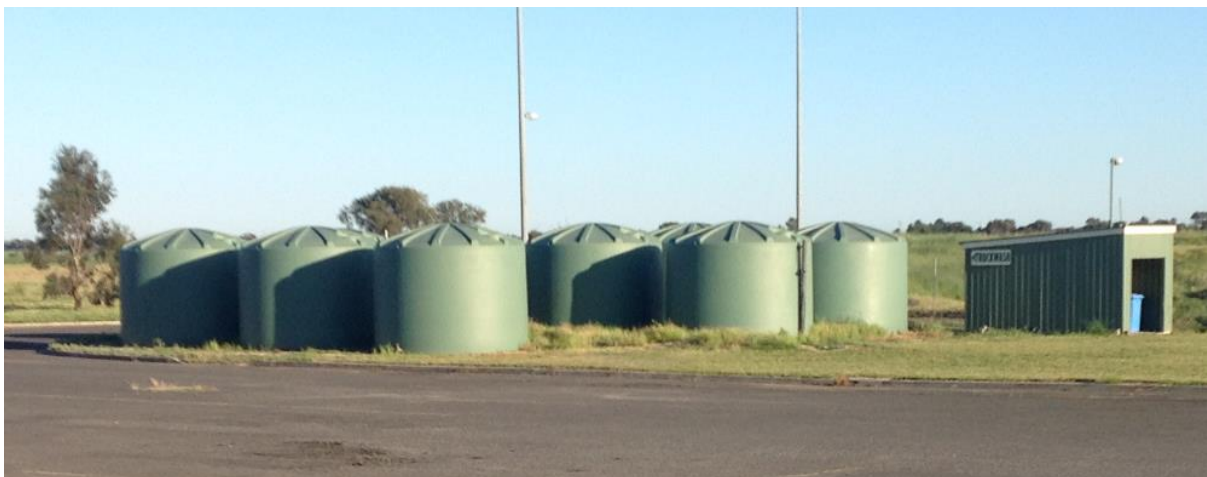
Water tanks for potable for drinking water and non-potable for washing water
