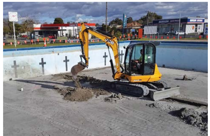
A $1.5 million refurbishment to the Horsham Aquatic Centre's outdoor pool was completed this year
