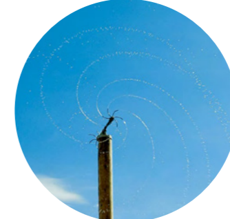
Spinning Pole-top sprinklers
