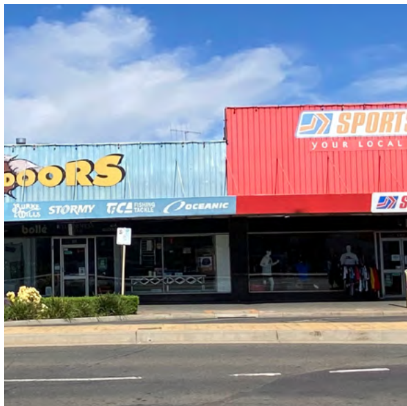
There is opportunity to remove metal sheet cladding where original parapets exist behind to reveal original detailing
