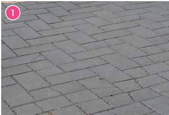
Concrete Paver Charcoal Herringbone Supplier: UrbanPave or equivalent Use: Main Footpath Surface
