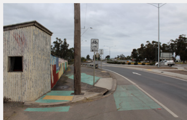
McPherson St near Stawell Rd intersection – Unprotected cycle access to off-road (shared) path. Kerb treatment not consistent with preferred cycle treatment.
