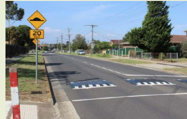
Speed cushions slow traffic at pedestrian and cycling crossing points.
