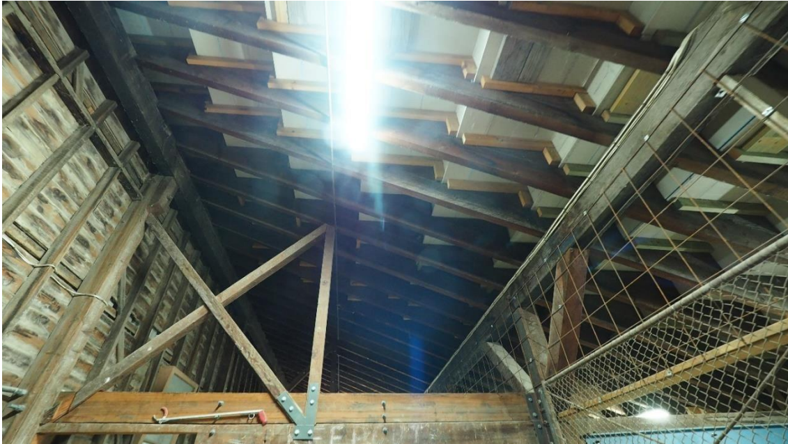
Figure 6: View underneath the grandstand seating (courtesy Stephanie Harder, Horsham Rural City Council)
