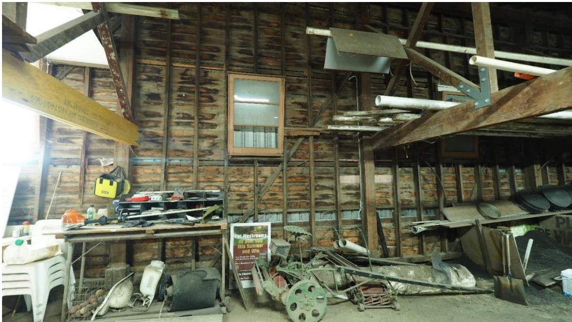
Figure 7: Under the grandstand showing old lining boards (courtesy Stephanie Harder, Horsham Rural City Council)
