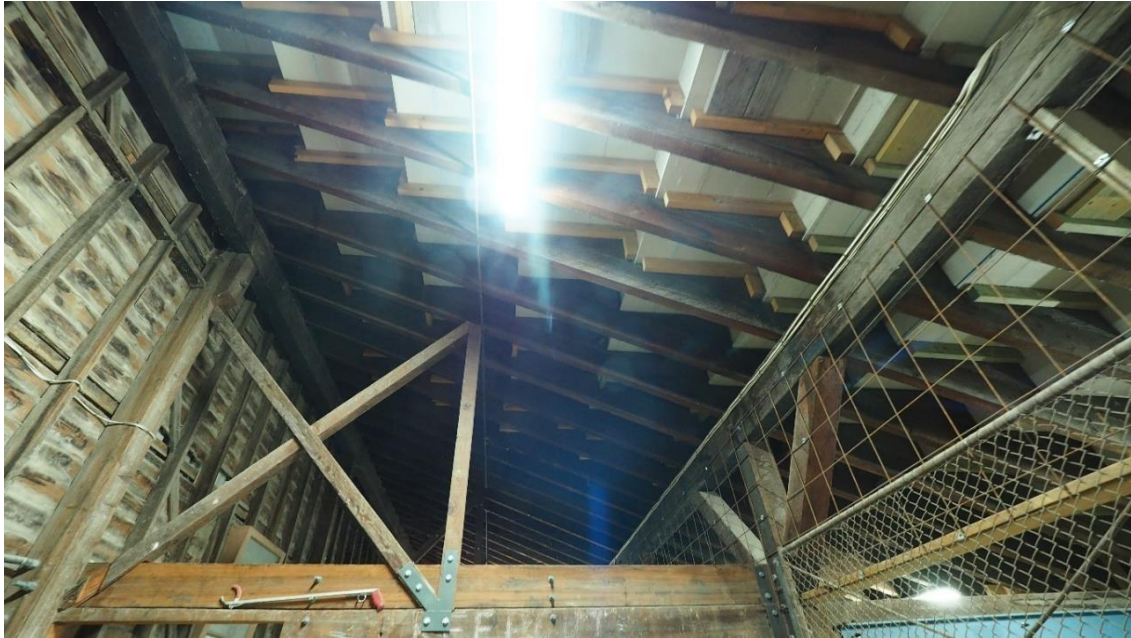
Figure 6: View underneath the grandstand seating (courtesy Stephanie Harder, Horsham Rural City Council)
