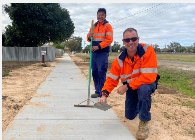
PAVING THE WAY: Urban infrastructure staff Johney Htoo and David Puls are pictured in Anderson Street where Council has this month constructed 400m of new footpath.
